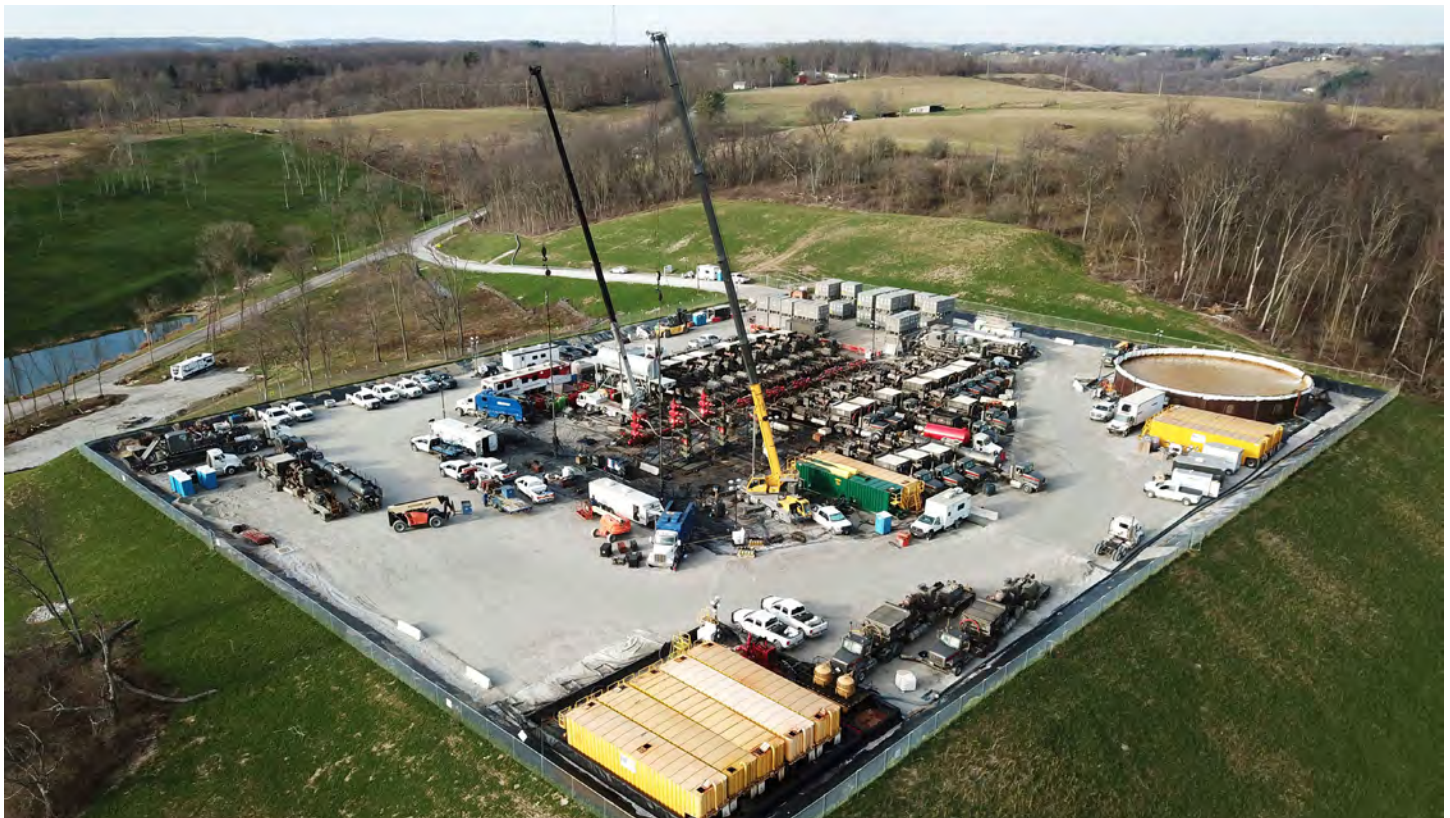
An aerial view of a frack pad site in Jefferson County, Ohio, in November 2020.
