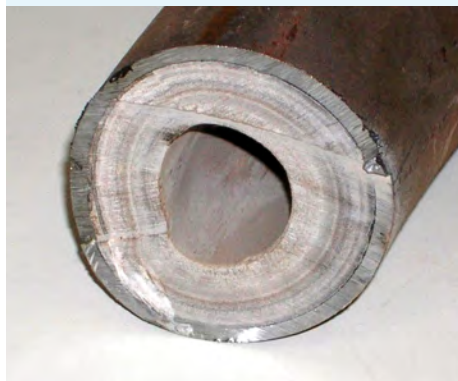
A cross-section of a heat exchanger tube with a thick layer of limescale build-up on the inner wall.
